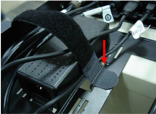
Figure 12: Power Supply Secured
